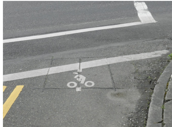
Pavement marking that indicates to bicyclists optimal positioning for signal detection.
